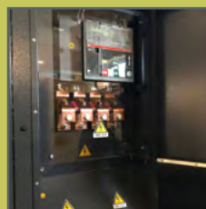
Connection copper bars for cables with lugs, they allow to connect more cables on the same phase
